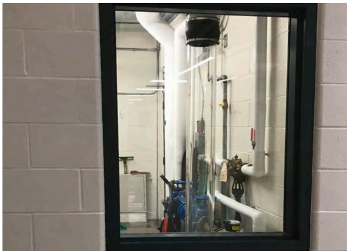
▲ A window allows students to see into the mechanical room.
