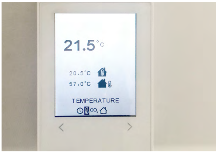
▲ An example of the controls provided to each classroom.
